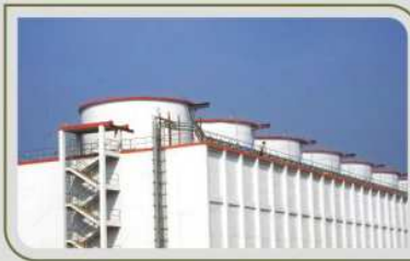
Concrete Cooling Tower
