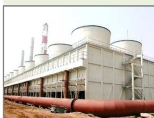
RCC CT (6 x 40000 m3/hr)
